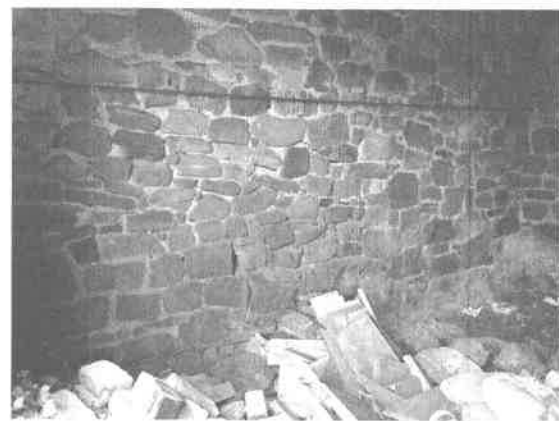
Image 10: Gaps between stone inside the lean-to structure.
