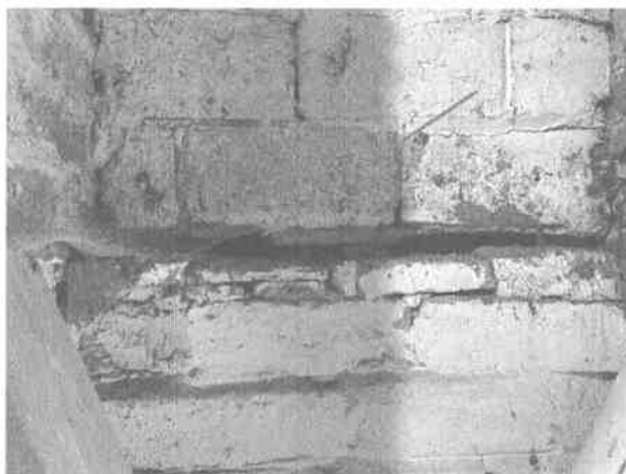
Image 9: Settlement crack in Barn 1.
