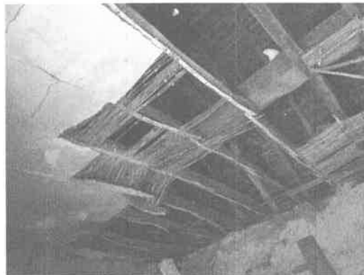
Image 6: Dilapidated ceiling in Barn 1 Section 2 of Barn 1.
