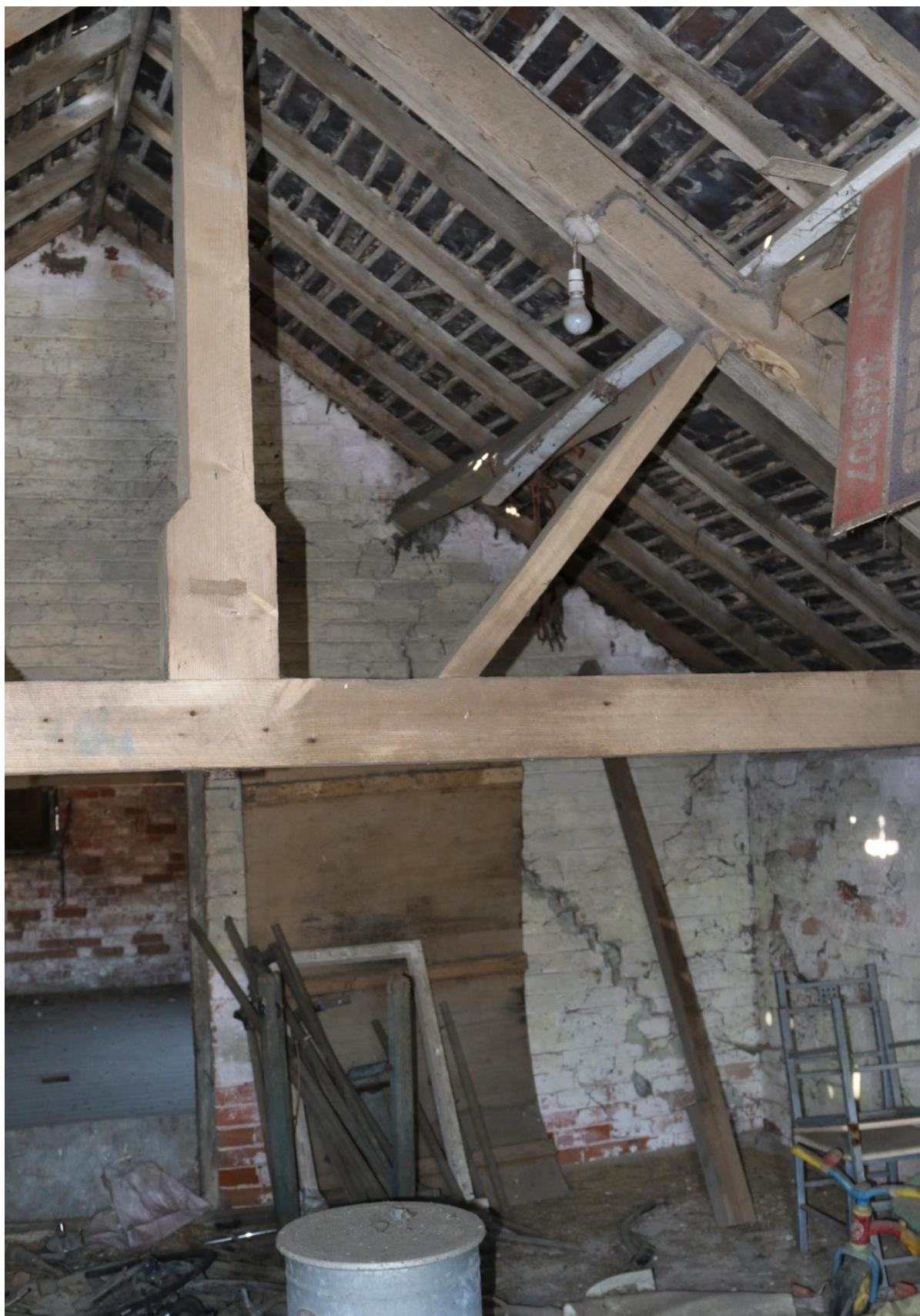
Image 9 – View from within the 1 st floor space which has demonstrated no membrane coverings below the roof tiles where several sections of protruding daylight was observed
