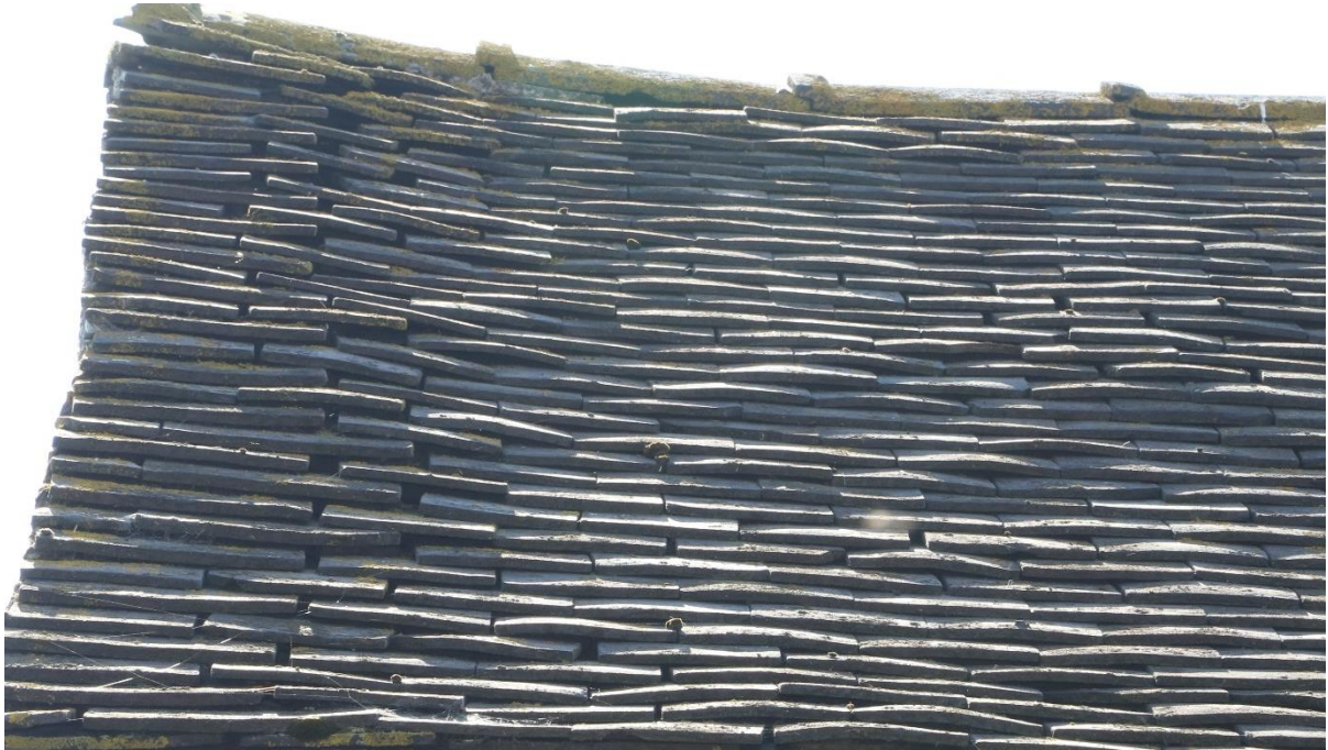
Image 3 – North facing roof coverings which have demonstrated moderate levels of movement/deterioration which may offer access & roosting values to bats within. Also gaps below the ridge tiles which offers a suitable roost environment for crevice dwelling bats
