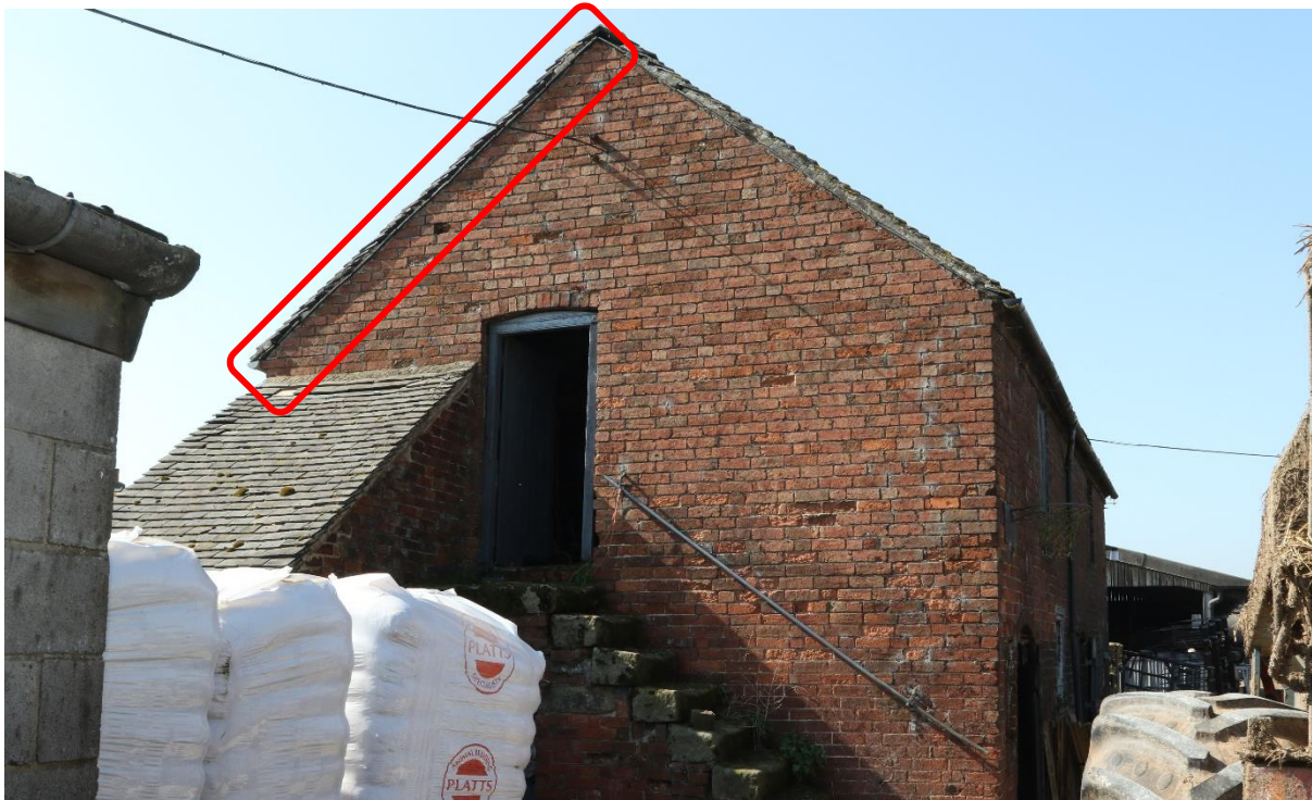
Image 4 – East facing elevation which offers a number of accessible crevices between the stonework's and roof coverings
