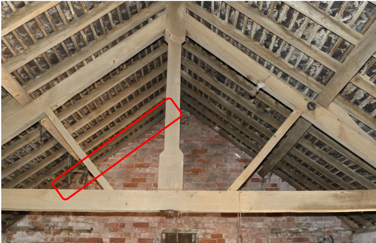
Image 10 – View from within the 1 st floor area to the far West of the building which has evidenced gaps between the roof coverings and stonework's which offers further value to crevice dwelling bats for roosting
