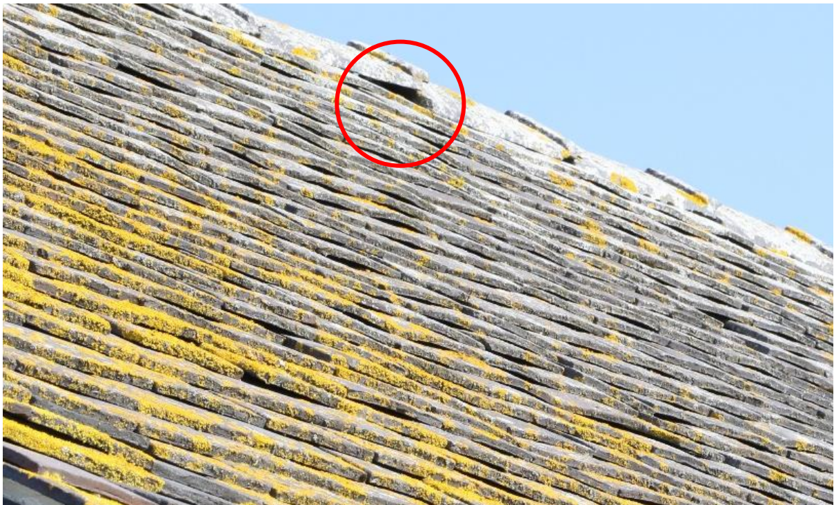
Image 6 – Gap below the ridge tiles within the South facing elevation which offers value to crevice dwelling bats within for roosting
