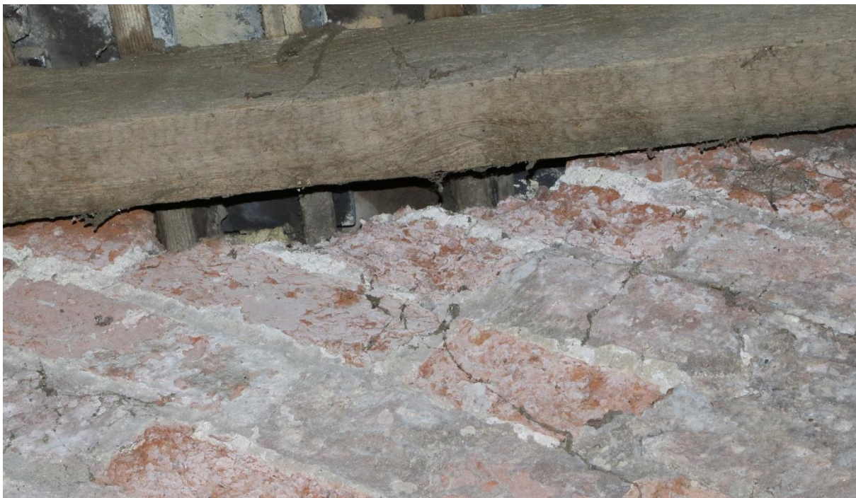
Image 11 – As image 10, gaps between the roof coverings and stonework's of value to crevice dwelling bats for roosting
