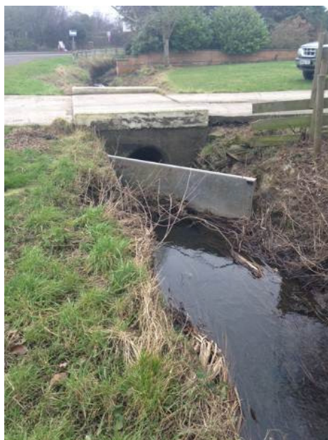
Figure 12: Picture illustrating baffle plate in channel
