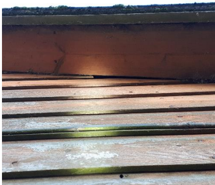
Photograph 3: B1 gap in soffit box
