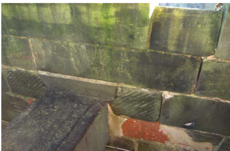
Fig. 23: View of one of the beam ends at the parapet abutment; cracking has occurred on both sides of the parapet and the felt covering around the beam casing has cracked/failed. The cracking and enlarged joints within the masonry are likely to have been caused due the additional weight of the modern steel structure used to strengthen the earlier timber beams. Image date 22 nd Nov. 2013.
