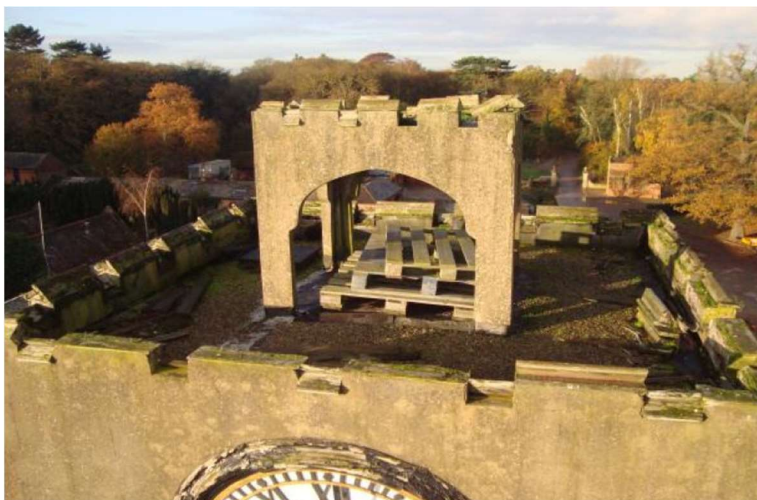
Fig. 22: View of the roof to the top of the Clock Tower & Belfry looking west. The roof has generally failed; several of the timber copings on the east side are missing leaving the asbestos cement board substrate exposed. Note; the Bell and weathervane are missing and the poor condition of the clock face. Image date 22 nd Nov. 2013.
