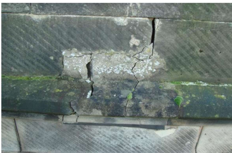
Fig. 24: Fracturing occurring to stonework moulding, with mortar patching to the end of the Clock Tower support beam on the west side at the south-west corner. This is most likely to have been caused by both the composite beams embedded within the parapet; the rusting steel channel and decaying timber. Image date 22 nd Nov. 2013.
