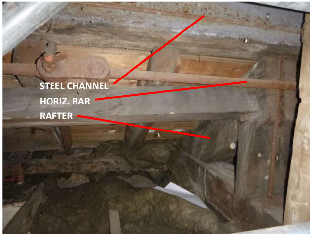
Fig. 18: Truncated principal rafter & timber support. Modern steel channels have been added, in addition to the earlier horizontal bar, to strengthen support to the Clock Tower structure. Image Date October 2016.
