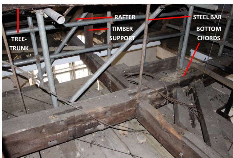
Fig. 17: Image from within the Clock Tower showing the bottom chords of the historic trusses. Note how an attempt to restrain these from sagging further has been made with the later central threaded steel tie-bar.; this is in turn supported inadequately by a tree-trunk which is just visible at the top of the image. One of the principal rafters, which has been truncated due to the addition of the Clock Tower, is just visible at the top of the image which is supported by a later timber post. Image date July 14 th October 2017.
