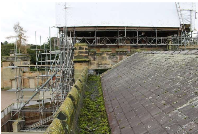
Fig. 20: Image from above the east range looking south of one of the Westmoreland roofs; all felt flashings and parapet gutters have failed causing water ingress problems. Image date February 2 nd 2017.
