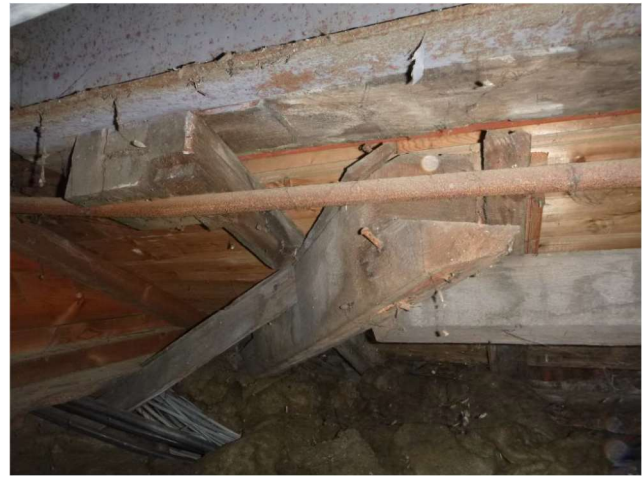
Fig. 19: Image of corner/hip rafter – note that the end appears to have been roughly sawn off to accommodate the clock tower structure. Image Date October 2016.
