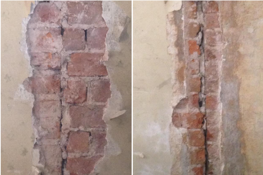
Figure 18 Straight joints visible internally (SW.13), July 2019
