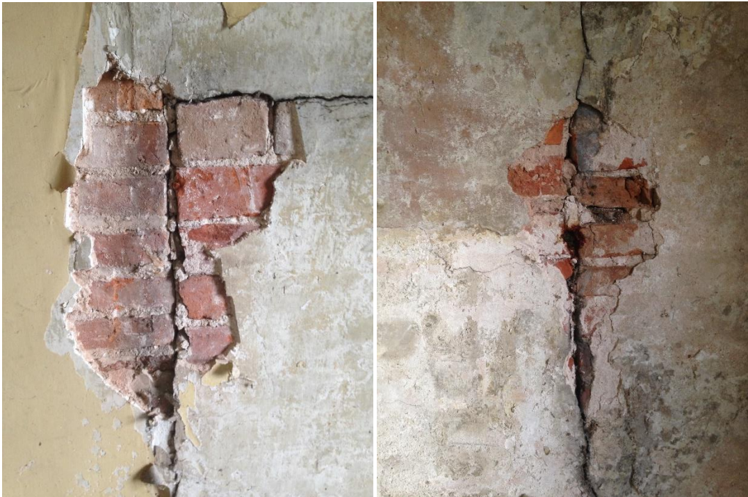
Figure 14 Straight joints visible at second floor (SW.08) July 2019
