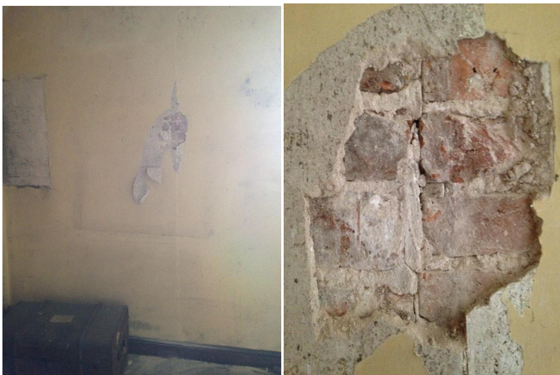
Figure 12 Straight joint visible internally at second floor (SW.05), July 2019
