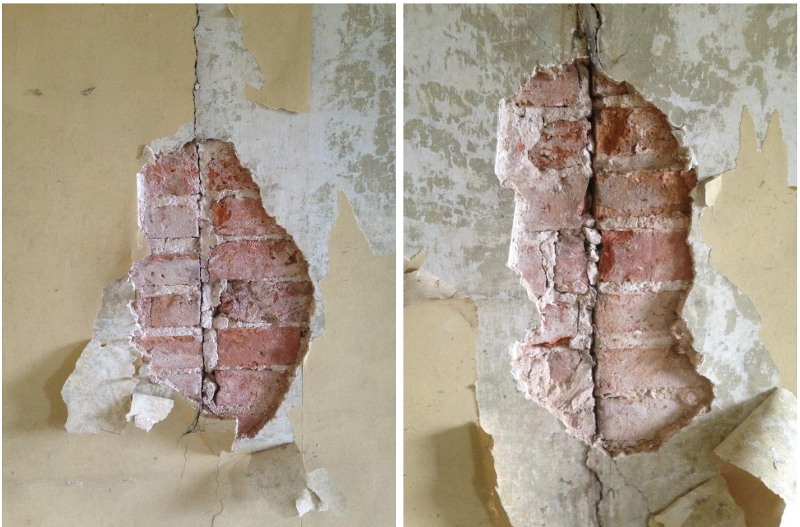
Figure 15 Straight joints visible at second floor (SW.09) July 2019
