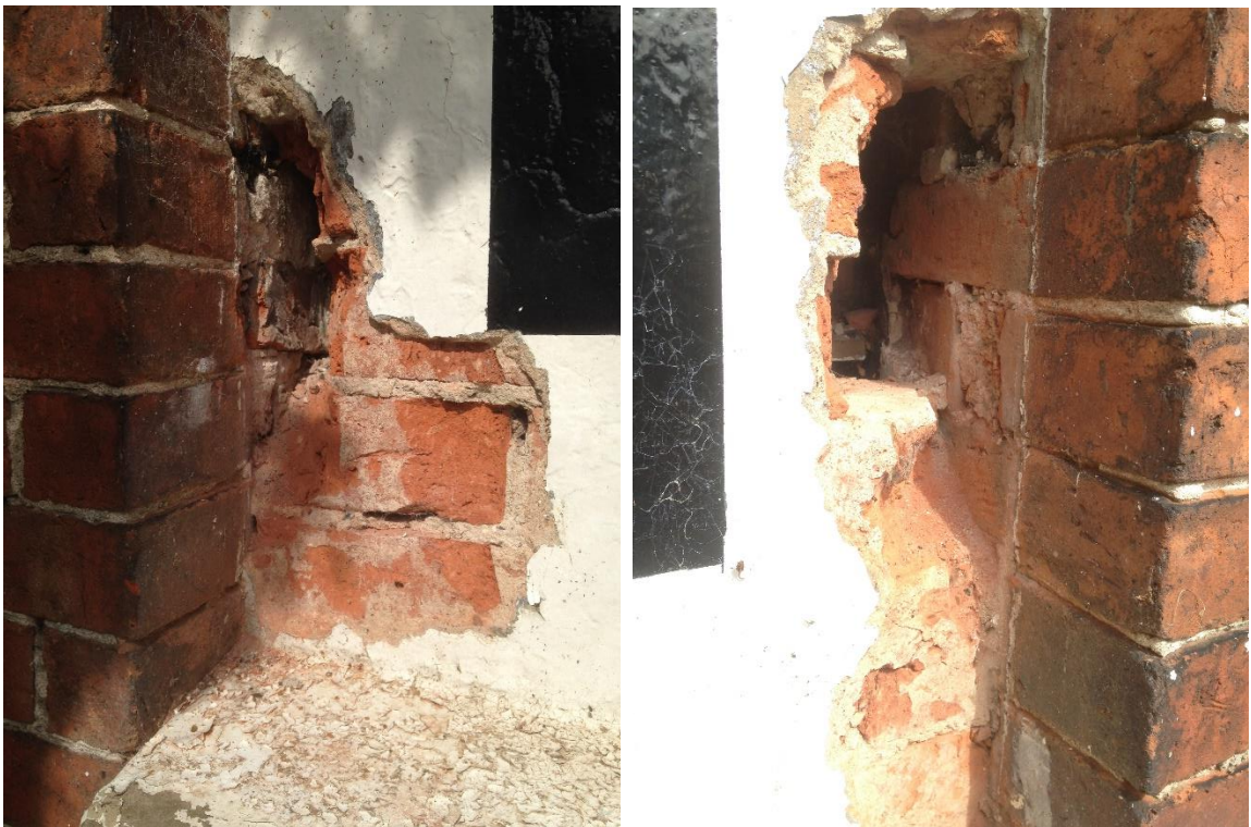
Figure 4 External opening up of render over infill of window GW.14 revealed that the coursing of the single skin brickwork between the reveals was different to that of the reveals, and was not toothed into it, suggesting it is a later infill of a previously existing window opening, July 2019
