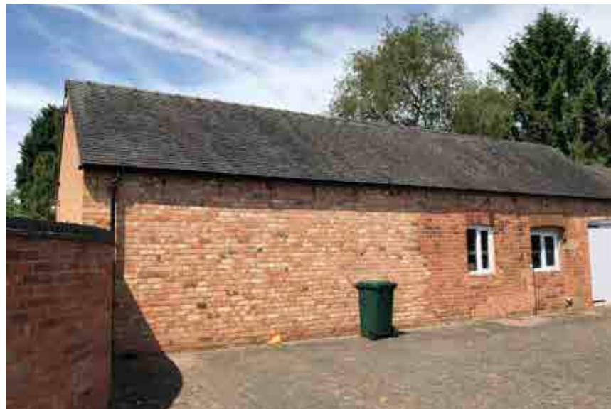
Evidence of previous extension and alteration to buildings
