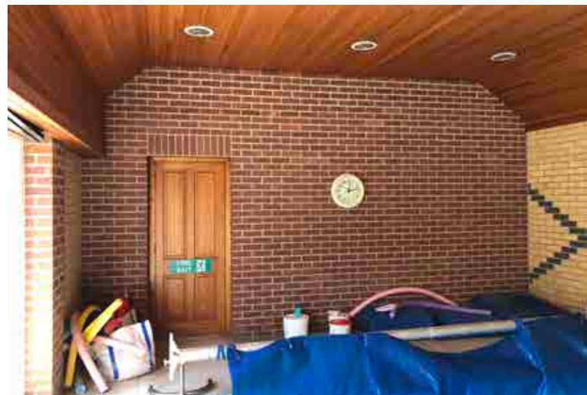
Unsympathetic modern materials used in previous alterations
