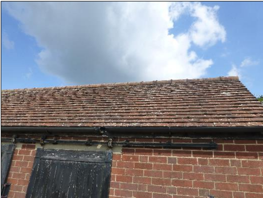
Photo 40. B14 – well sealed
