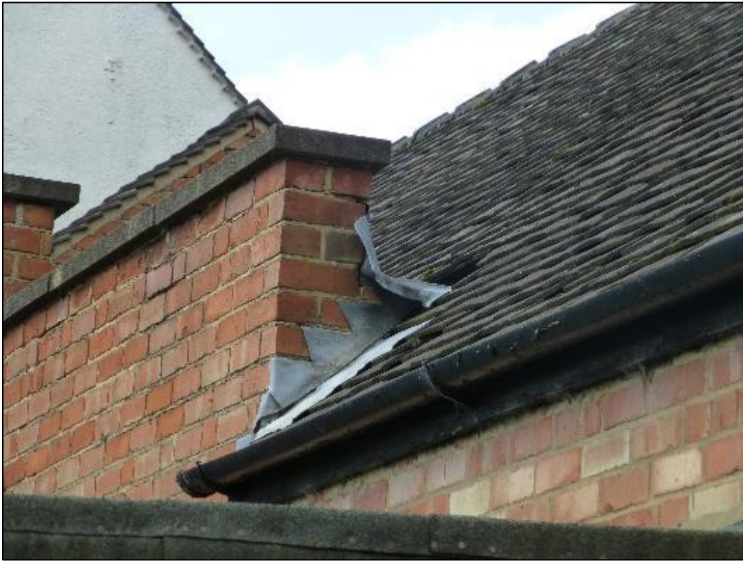
Photo 29. B9 – gaps below tiles / led flashing
