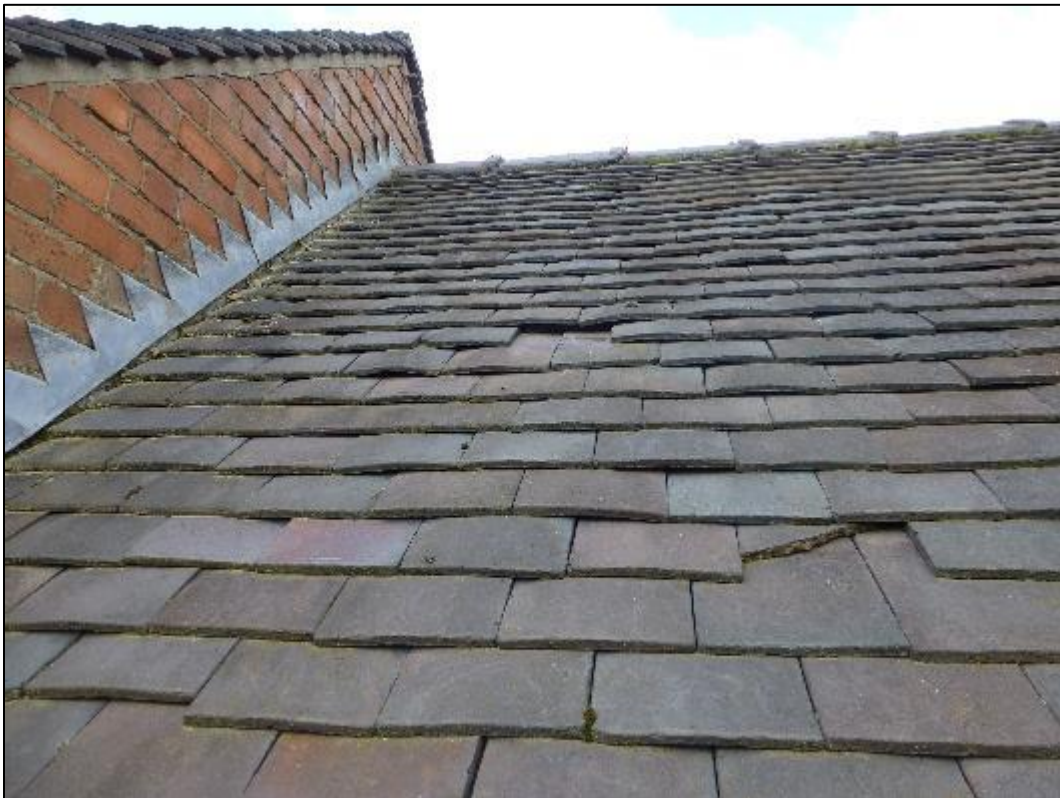
Photo 24. B7 – gaps below tiles
