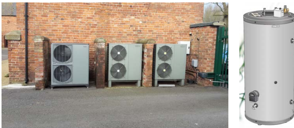
Figure 7 Typical external ASHP units in-situ (42kW) and internally located hot water cylinder (500l)
