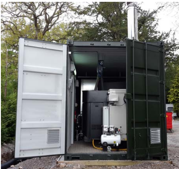
Figure 6 Containerised biomass boiler with integral flue
