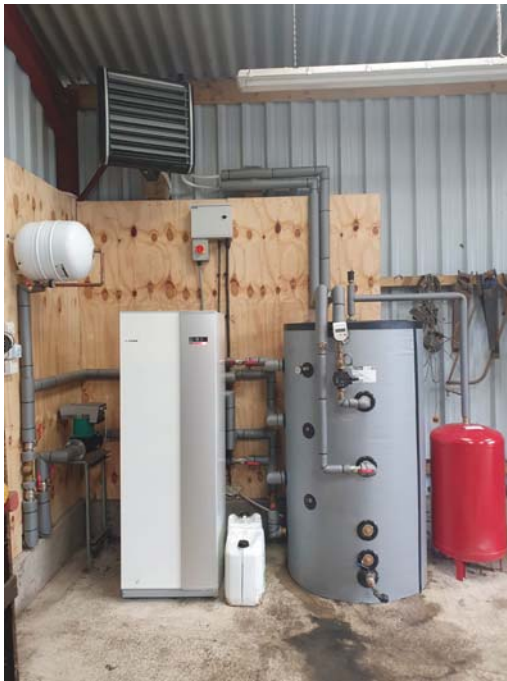
Figure 8 60kW ground source heat pump in a plant room. Shown alongside a thermal store with associated pipework
