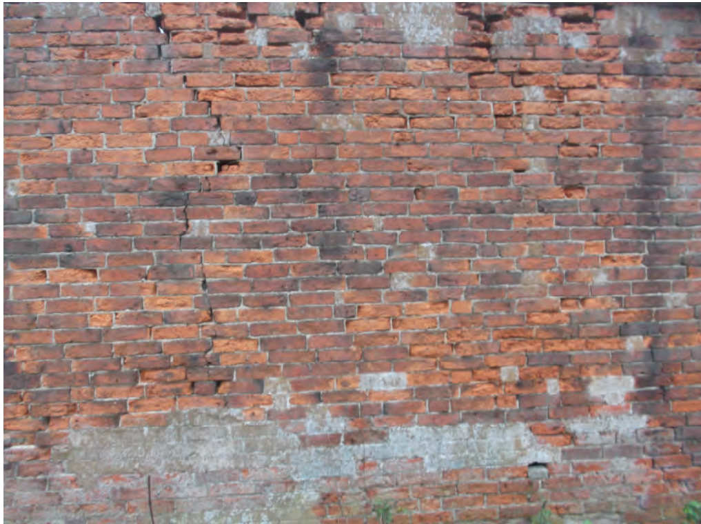
Photograph 6 – Wall E mid-way between junctions with walls D and C – vertical crack and point at which wall can be rocked.
