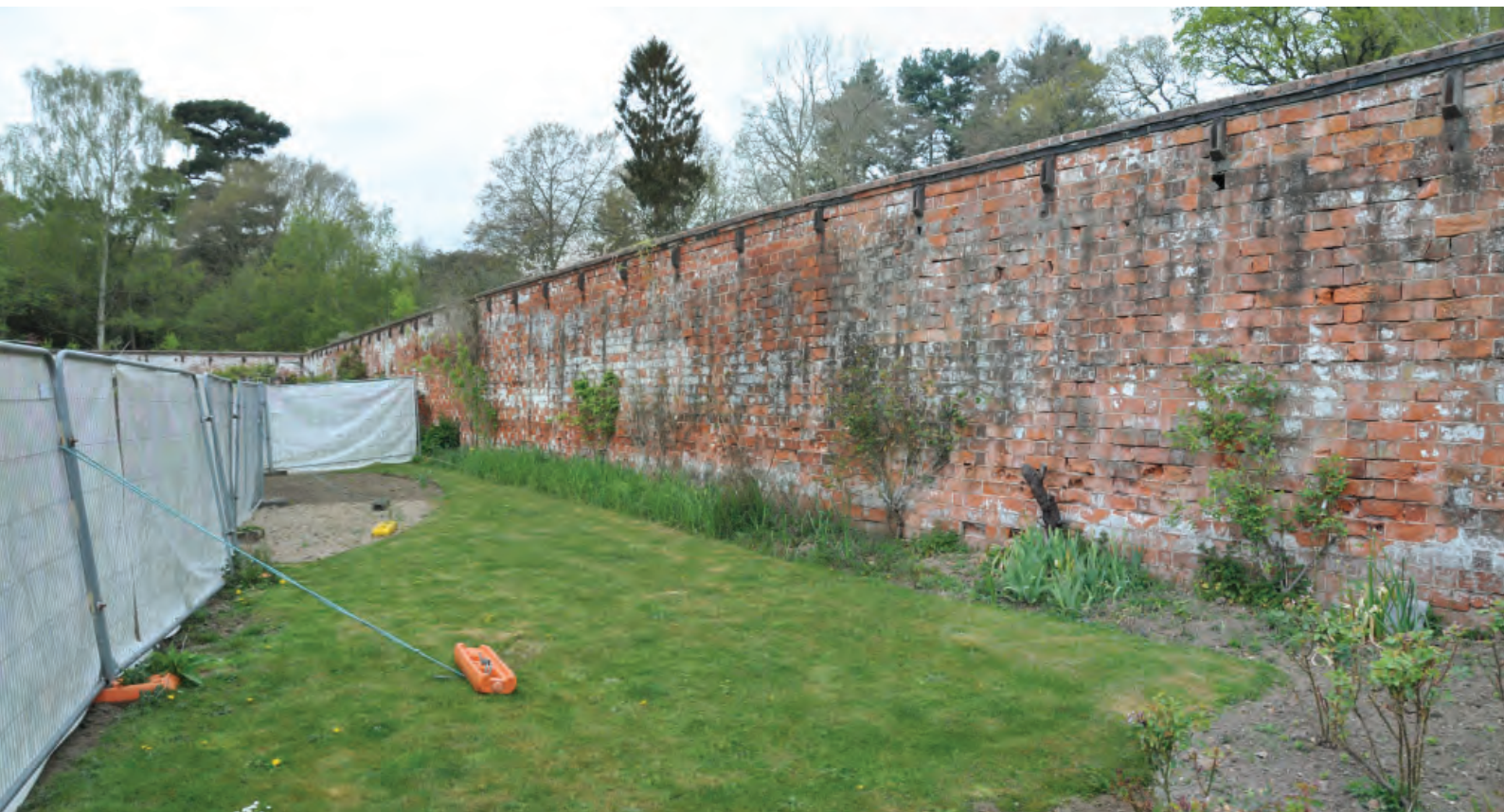
Fig. 8 (above): Panoramic view of south elevation of the heated wall (facing west); note the presence of further areas of missing and badly eroded bricks along its length.
