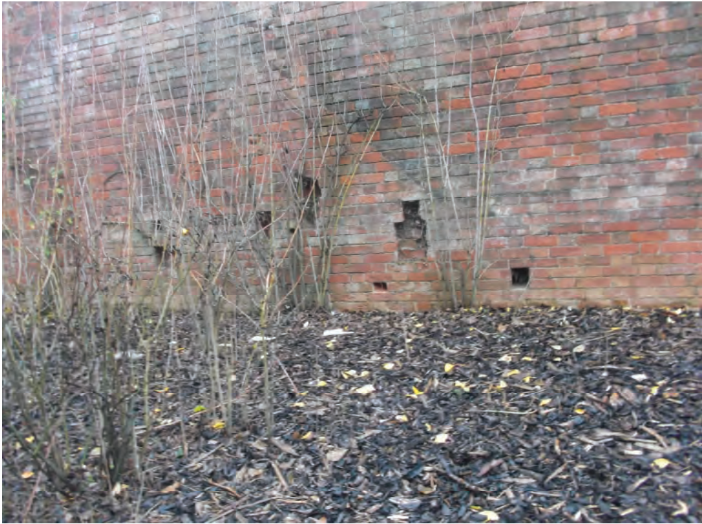
Photograph 4 - Wall B - west side- missing bricks in wall.
