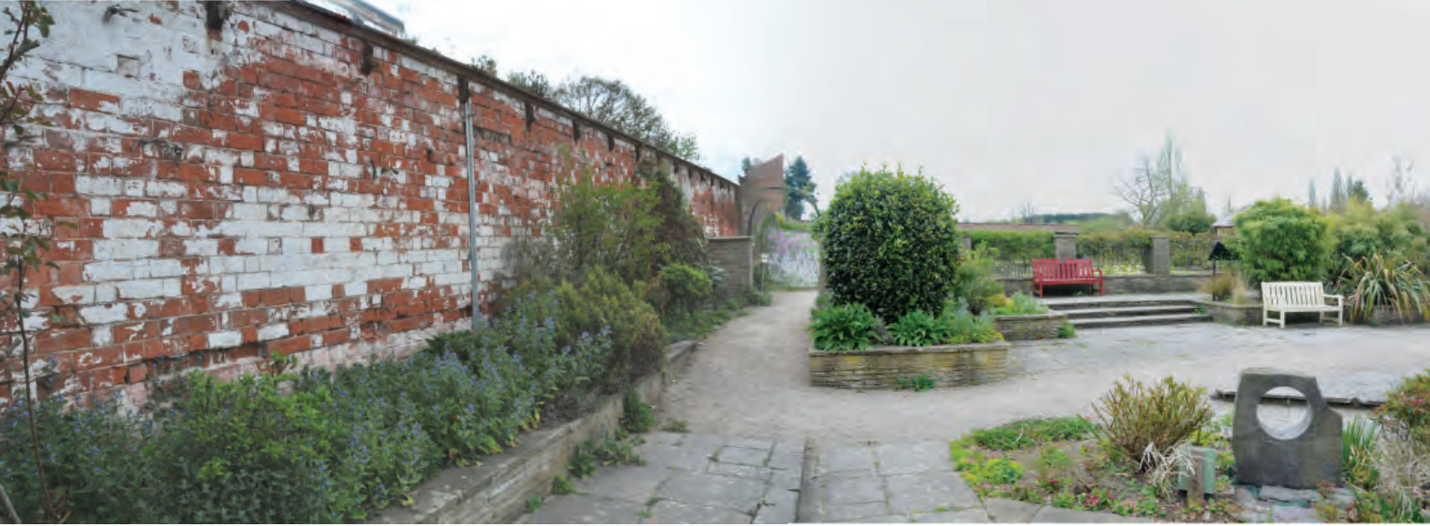
Fig. 7: Panoramic view of south elevation of the heated wall (facing east); note the poor condition of the wall with multiple missing areas of brickwork. The wall is to be rebuilt along its entire length to the same height, proportions & materials.
