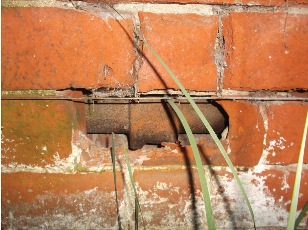
Photograph 1 - Wall A - cast iron heating pipe within cavity
