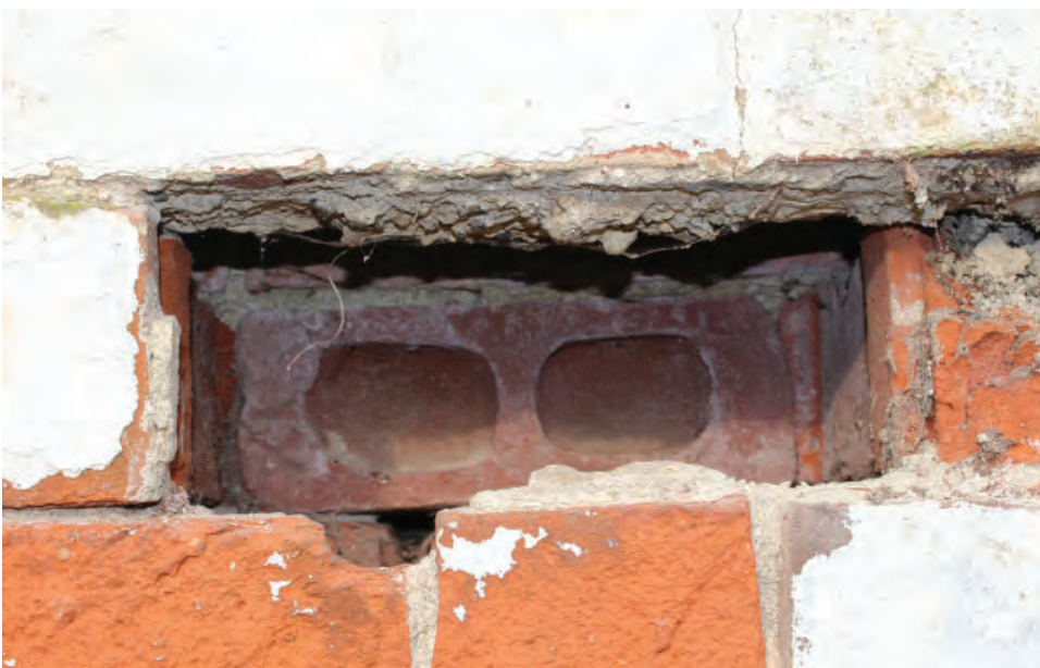
Fig. 15: A further, existing, hole in the wall approximately 1.8m above ground level where the inner face of the cavity wall is visible. A double-frogged brick is clearly visible, a type which appear to have been used exclusively within the interior wall.
