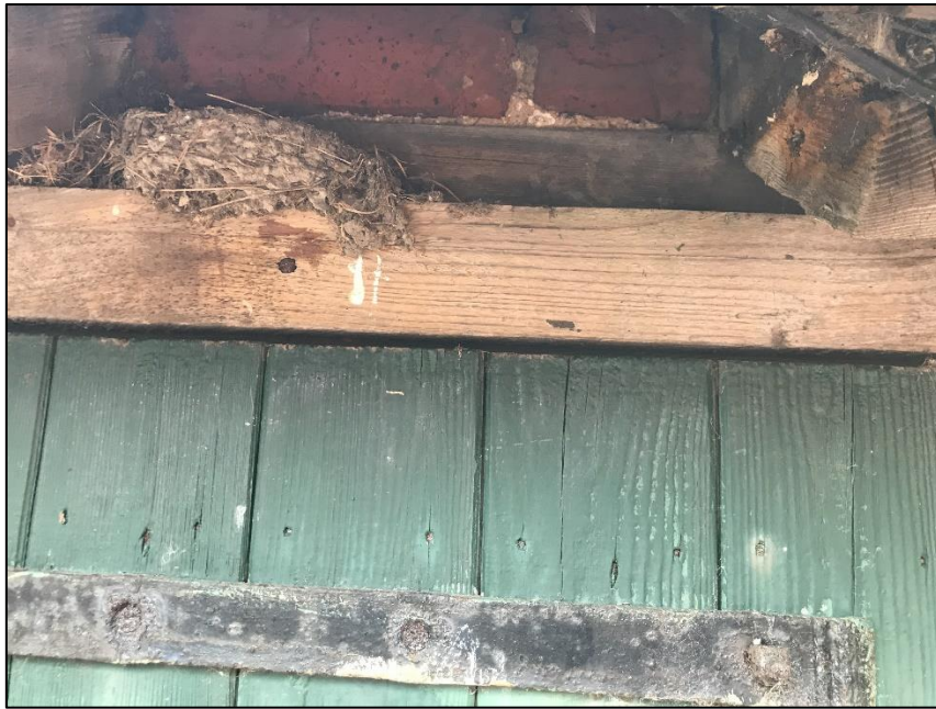
Plate 7. Swallow nest located above double barn door on the northern aspect
