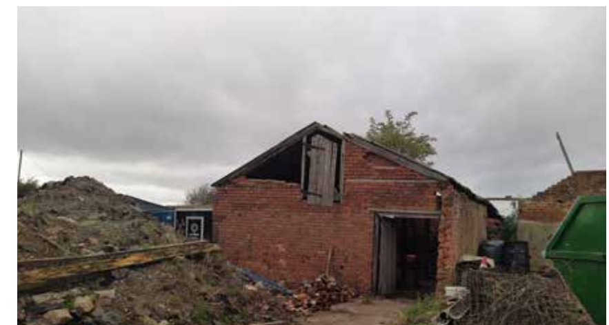
Remains of detailing on the Games Room barn
