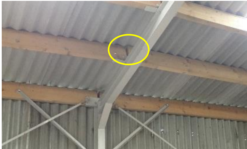
Photograph 6: Gaps between timber beams in middle of roofing frame
