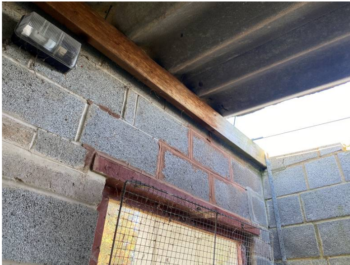
Figure – timber lintel over window and local re-pointing. Note exposed to elements due to broken roof sheeting
