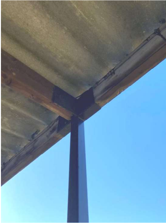
Figure – corrosion to top of column brackets
