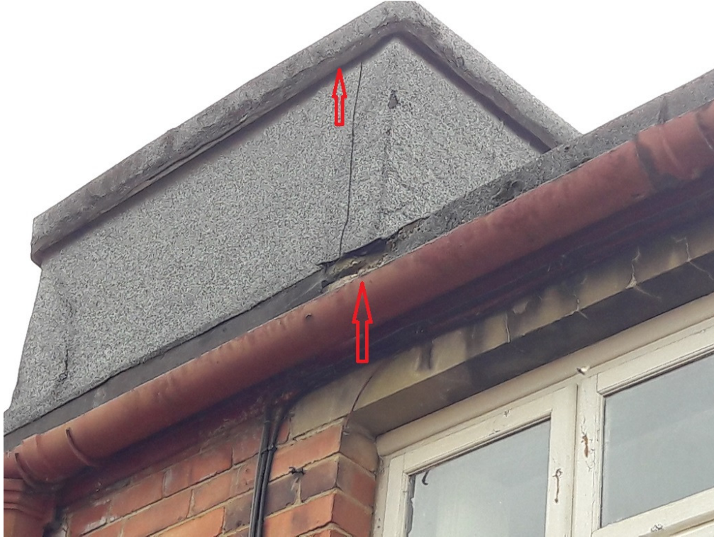
Photos: potential access points where roof felt damaged and on box structure (indicated by red arrows).
