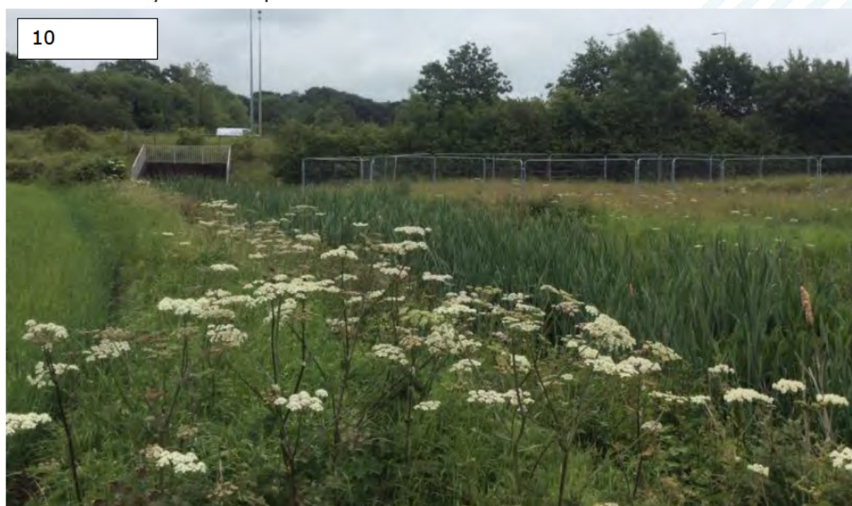
Figure 2-8: Over-wide channel upstream of road bridge culvert
