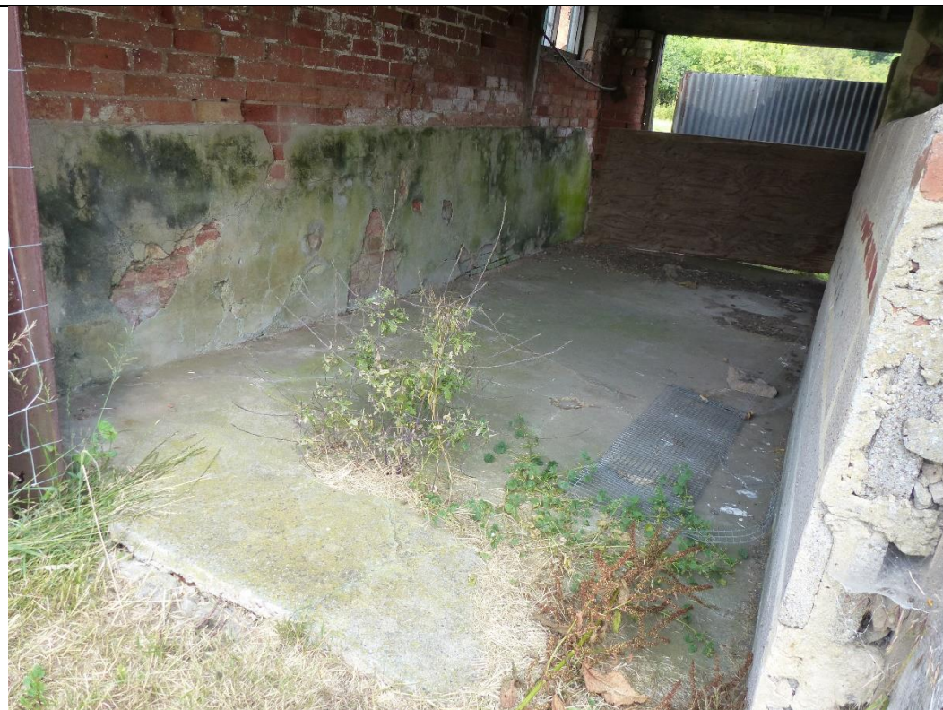
Photo 12 – Barn 2 – Failure of concrete floor slab and internal render causing external damp issues
