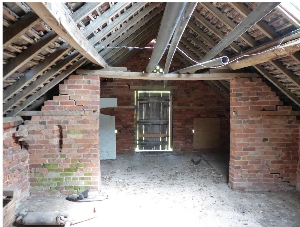
Photo 6 – Barn 1 – Deflection of main roof / failure of internal load-bearing masonry walls
