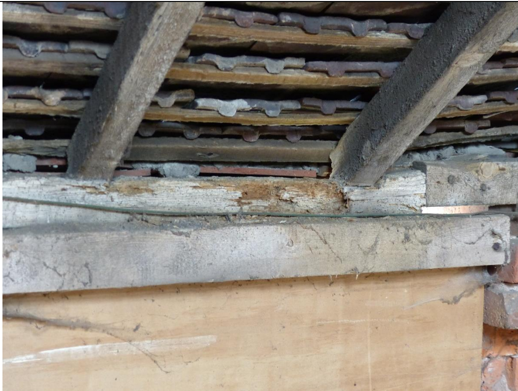
Photo 7 – Barn 1 – Beetle infestation to timbers
