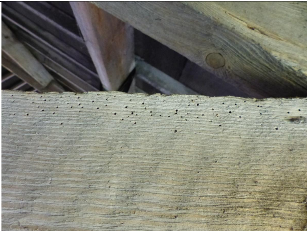
Photo 14 – Barn 2 – 'Flight' holes noted to King post truss bottom cord and timber wall plates
