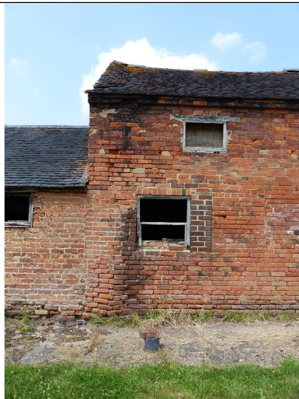
Photo 4 – Barn 1 – Failed Masonry Wall
