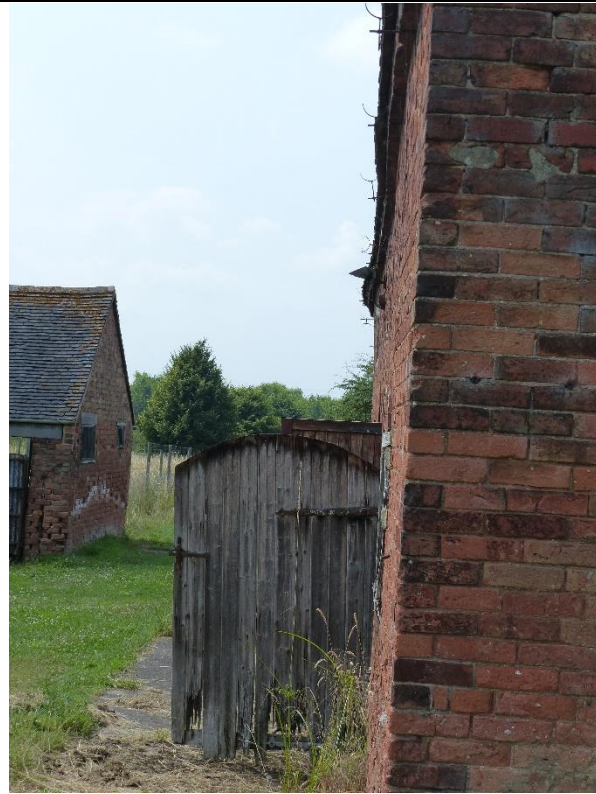
Photo 3 - Barn 1 – Undulation to roof / eaves brickwork course due to 'roof spread'
