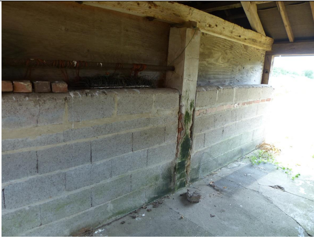
Photo 13 – Barn 2 – Failing brickwork pier supporting King post trusses
