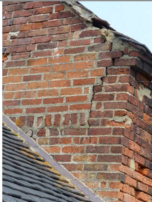
Photo 5 - Barn 1 – Failure of gable end / roof junction
