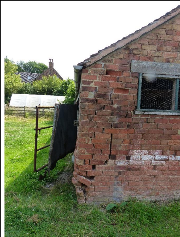
Photo 9 – Barn 2 – Failure of brick pier
