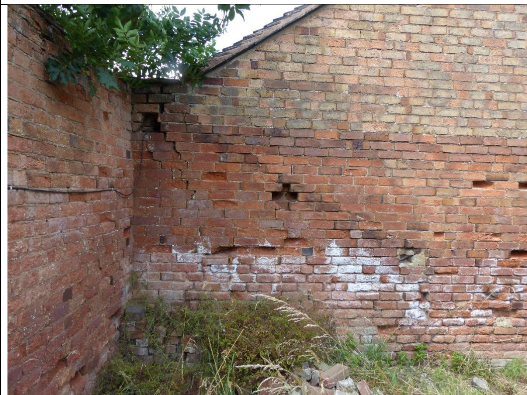
Photo 10 – Barn 2 – Failure of brickwork due adjacent ash tree and brick spalling / salts
