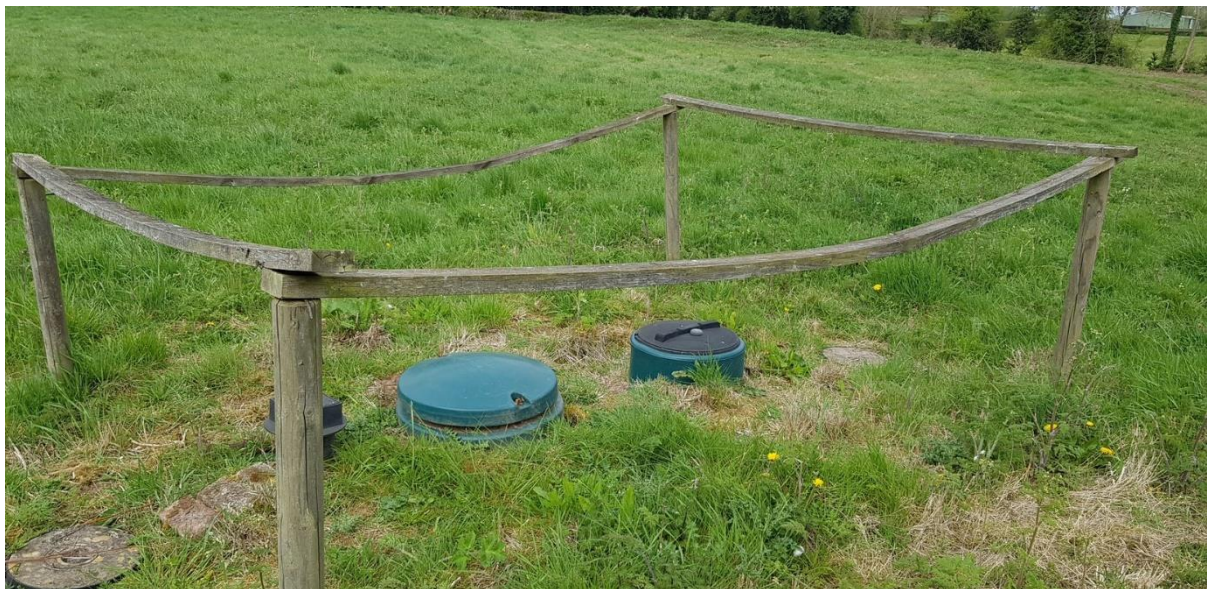
Photo 16. Modern in-use septic tank.
