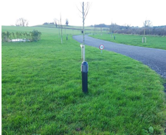
Photo 3: Light bollards both side of new road.
