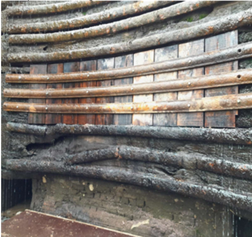
Plate 60 – example of similar fendering installed at Stenson Lock
