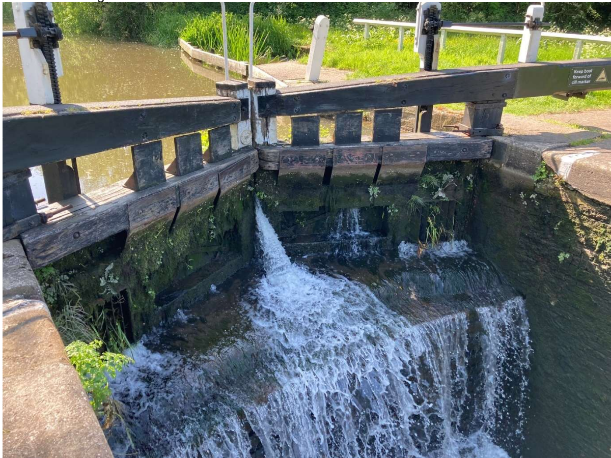
Plate 50 – leakage at cills
