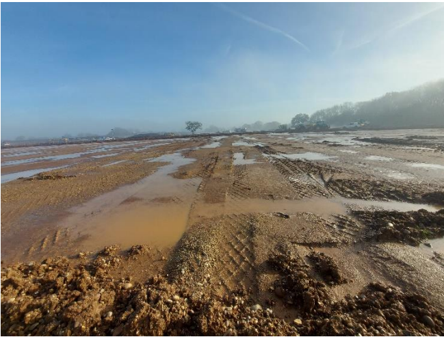
Z4 towards east – Ponding water observed across the development platform, mostly frozen.
