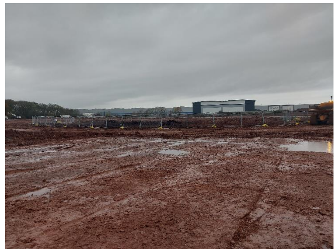
R11 towards S9 – Marl pit area has been fenced off following the discovery of asbestos and other potential contaminants.
