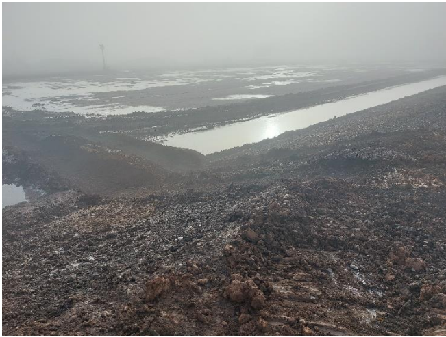
P3 towards South – Ponding water within the development platform – frozen at certain locations.
