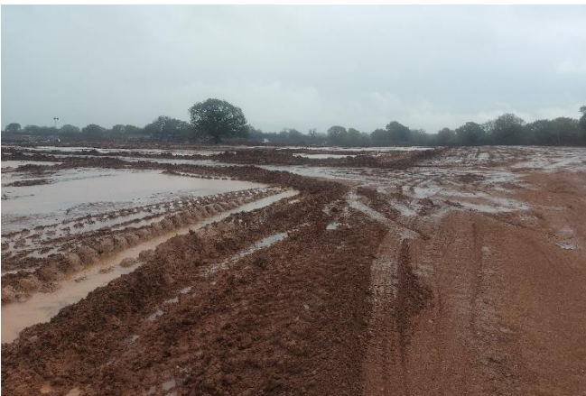
Z5 towards East – Ponding water across the development following the morning rain.
