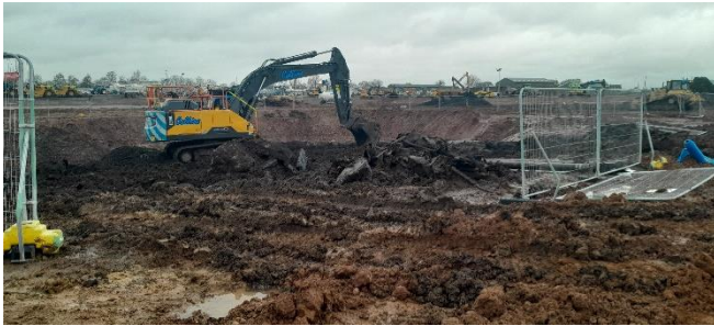
Grid R;10 towards Northwest – Riddled unsuitable materials.
