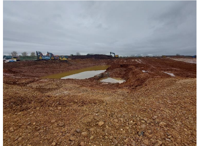
M6 towards North – Infilled Pond in the northern part of site is fully excavated – ponding water is noticed.
