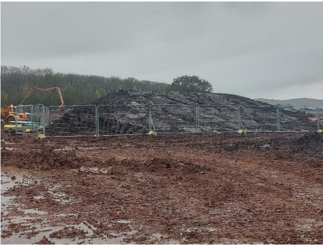
S12 towards U11 – Potentially contaminated subsoil material from the Marl Pit has been stockpiled, isolated, and securely fenced off following the discovery of asbestos and other suspected contaminants.
