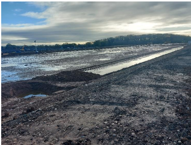
P3 towards South – Ponding water within the development platform.
