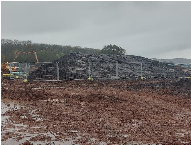
S12 towards U11 – Potentially contaminated subsoil material from the Marl Pit has been stockpiled, isolated, and securely fenced off following the discovery of asbestos and other suspected contaminants.
