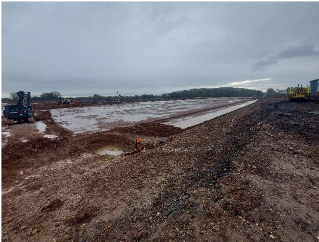
P3 towards South – Ponding water within the development platform.
