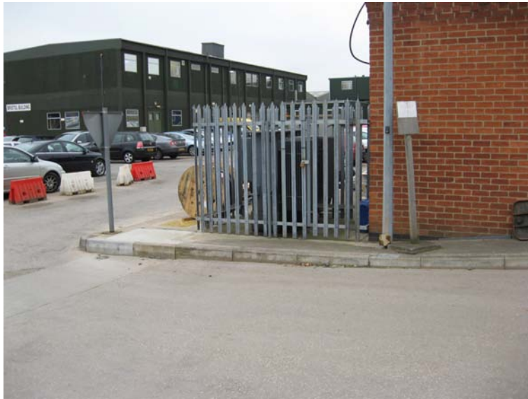
Plate 25: Substation in central area of site
