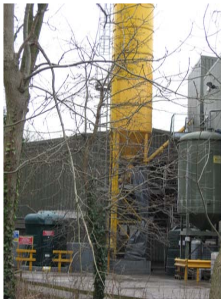
Plate 2: Silos, IBC's and other site chemical storage in site
