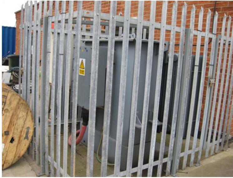
Plate 26: Substation in central area of site
